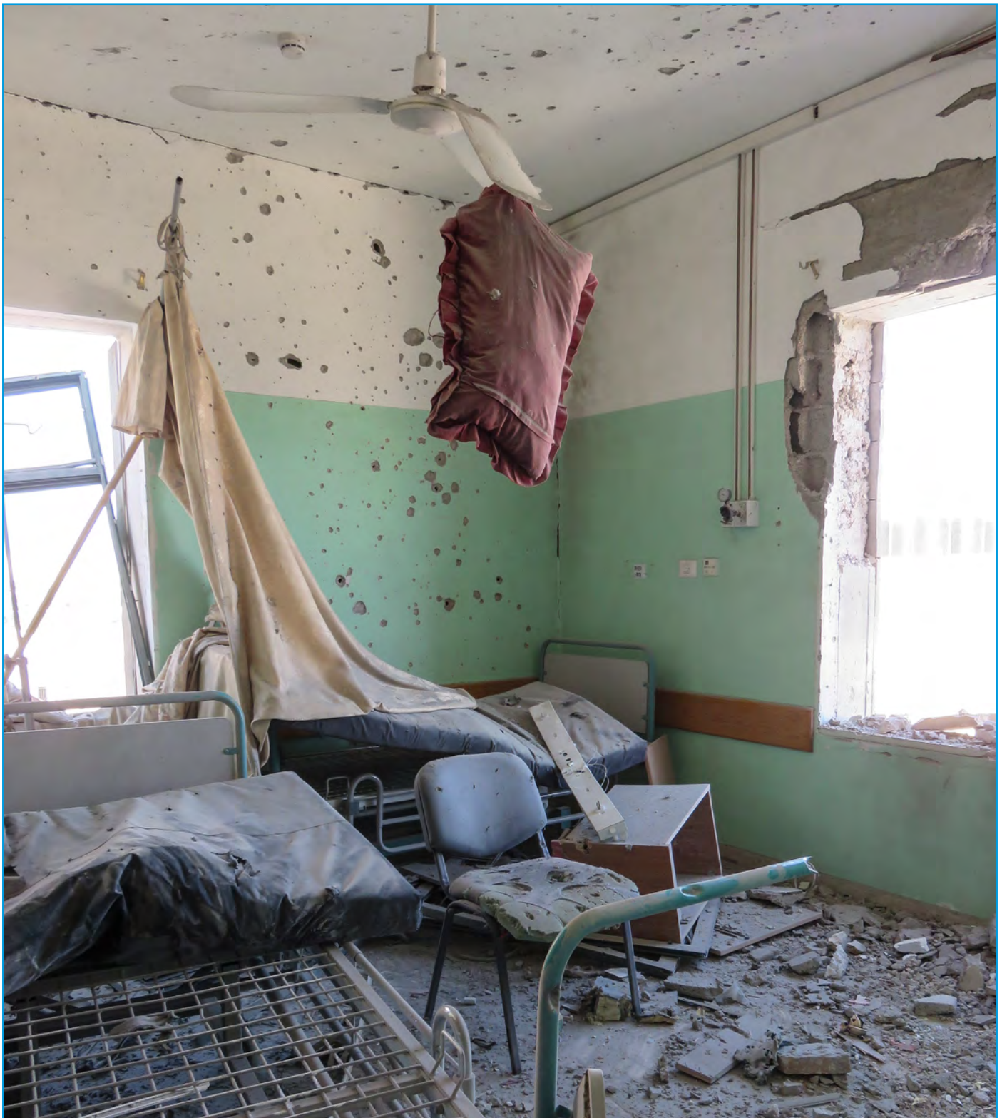
Gaza city, Al Aqsa hospital damages caused by shellings. @ICRC
